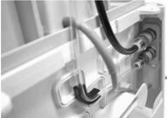
Fig. 6.3.4.12: Connection of power cable, AWS & flushing
